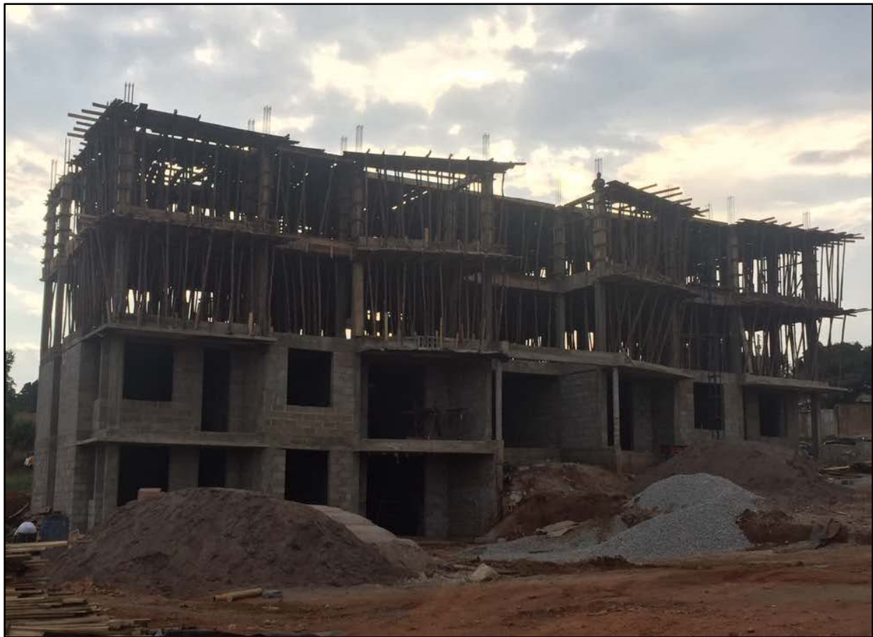
In this photo taken in mid-March, construction of the Gary S. Holmes Residence is well under way. The Susan and Thomas Bisanz Residence and the Megan and Dennis Doyle Residence soon will follow.
